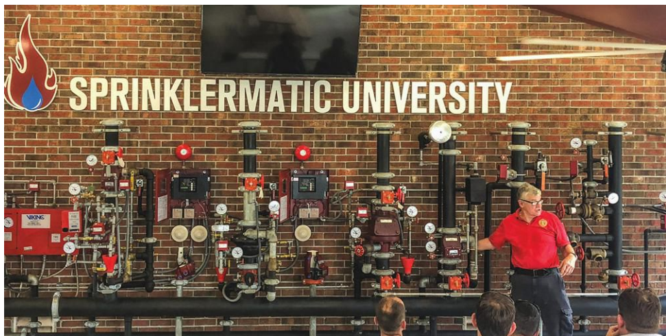
Miami-Dade Fire Rescue Captain Bill Gustin walks firefighters through a variety of risers at the onsite wet lab.
